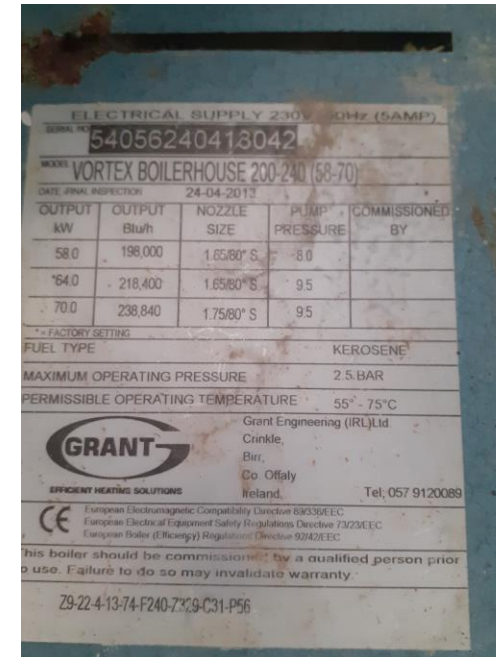
Current heating system- 2 x 60 KW oil boilers
